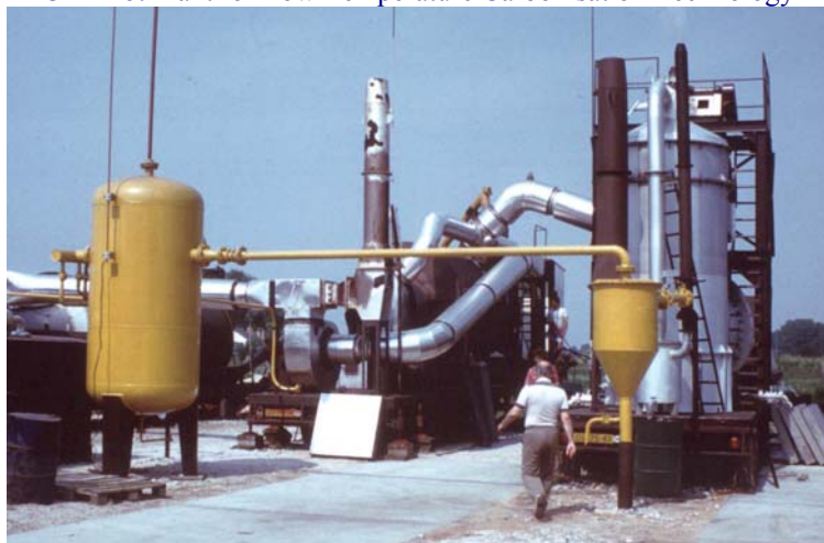
3R Pilot Plant for Low Temperature Carbonisation Technology
